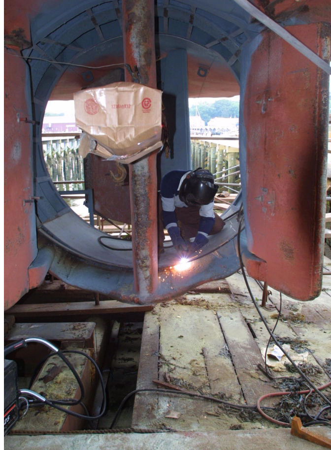
Foss Shipyard Welder Think Tien Nguyen repairs the kort nozzle on one of Constellation’s tugs. He and another Seattle welder traveled to Gloucester, Mass., to perform the work.
