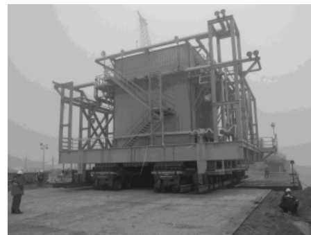
One of the first modules delivered to Sakhalin Island this summer rolls off the barge.
