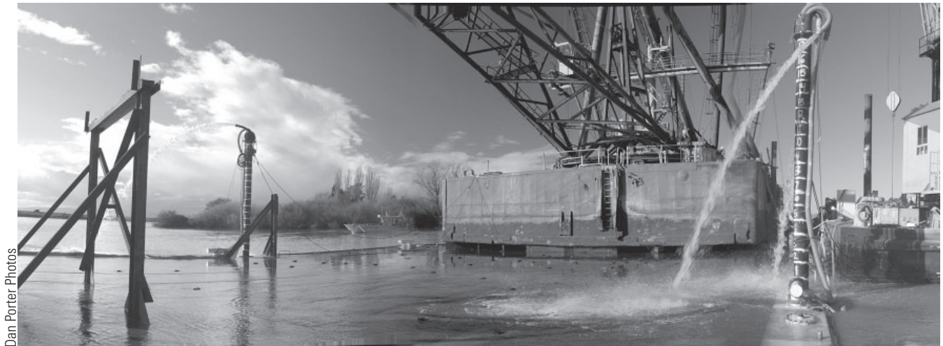
The deck of the submersible barge MZB287, with the Monarch on board, breaks the water as the pumps run full tilt.
