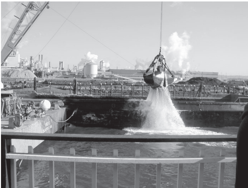
A clamshell dredge is at work in this photo taken from the porch of the Foss Tacoma office.
