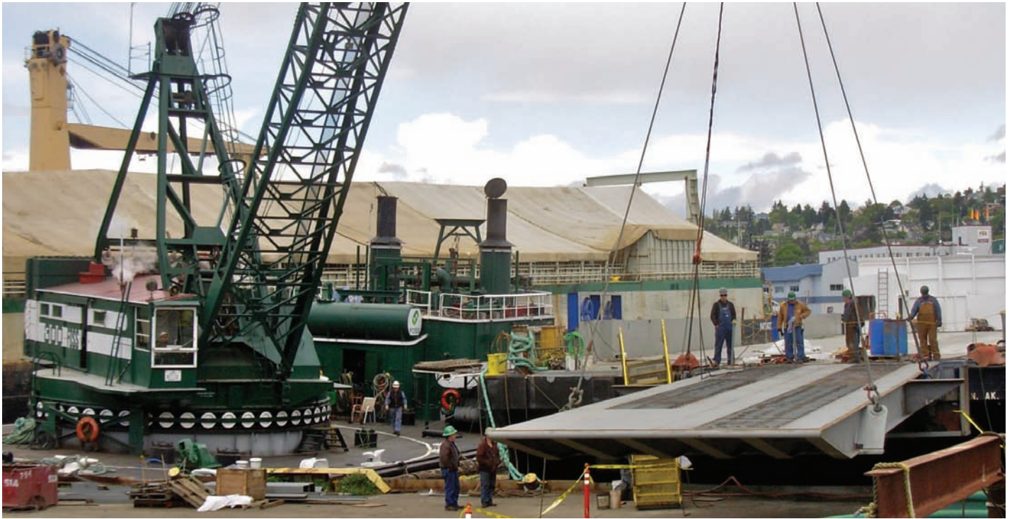
The Foss 300 derrick lowers a new ramp into position on the barge Spruce , owned by Olson Marine,
