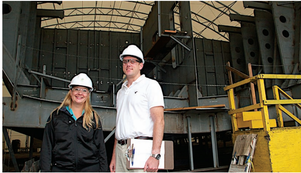
Erika Weber and Matt Baker have been working overtime to keep up with the Long Beach fireboat project. Behind them is the midsection of the hull.
