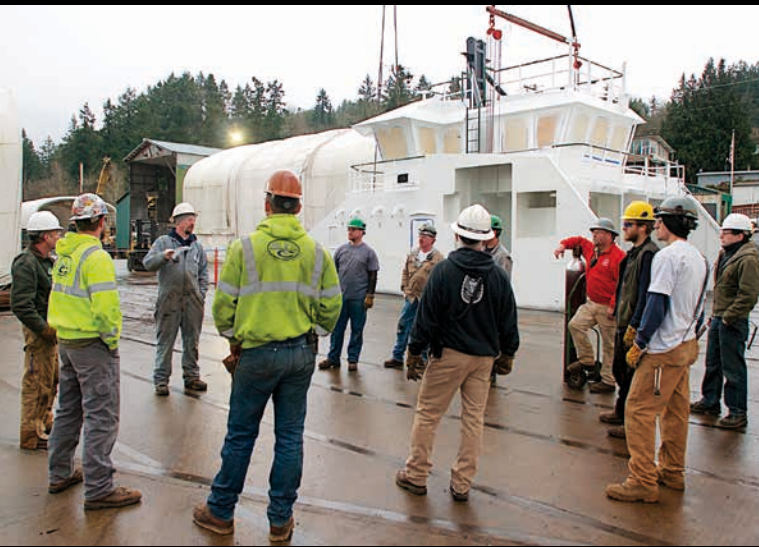
▲ Above: Project Foreman Corey Cook , facing the camera in coveralls, led a safety meeting before the pilothouse was lifted from the ground.
