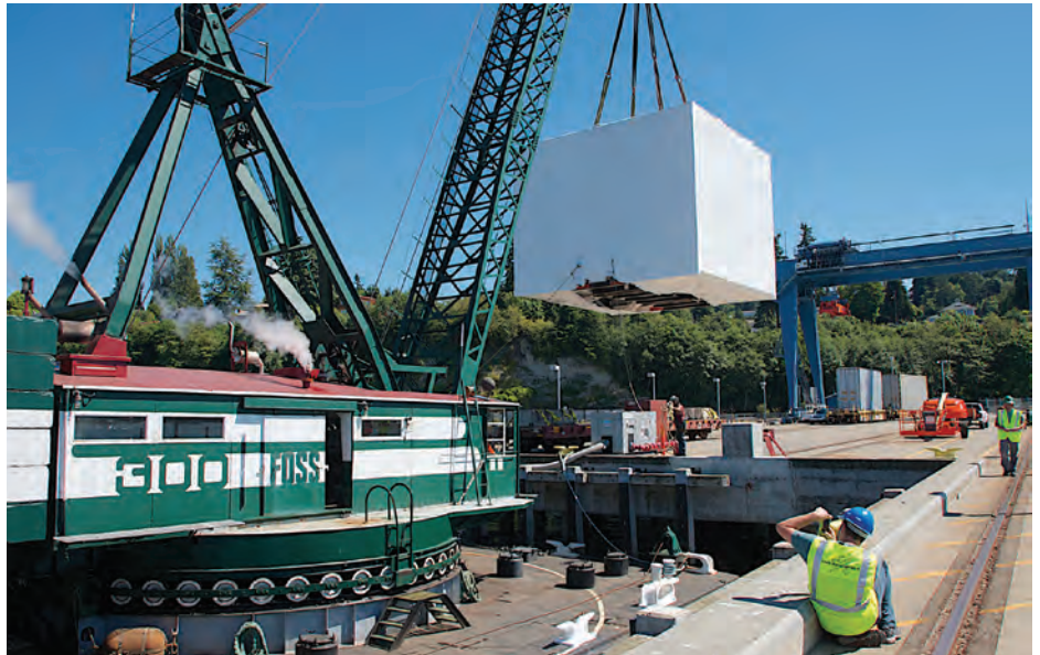
The Foss 300 derrick lifted the bulky package holding the riveting machine from a rail car before moving it to the barge 185 C-3, which was waiting a few hundred yards offshore.
